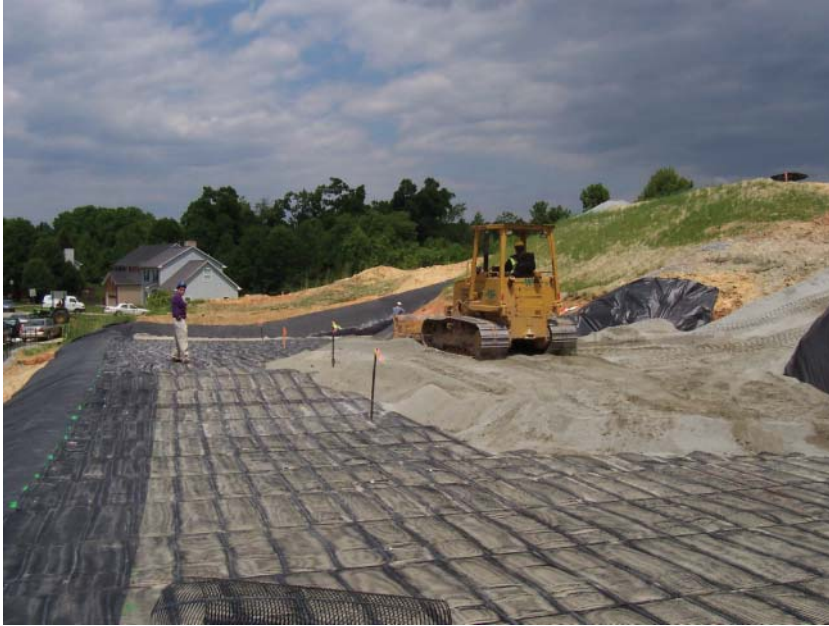
Fig. 8.11 Example of a reinforced soil slope in construction. (Photo courtesy of Tensar International.)
