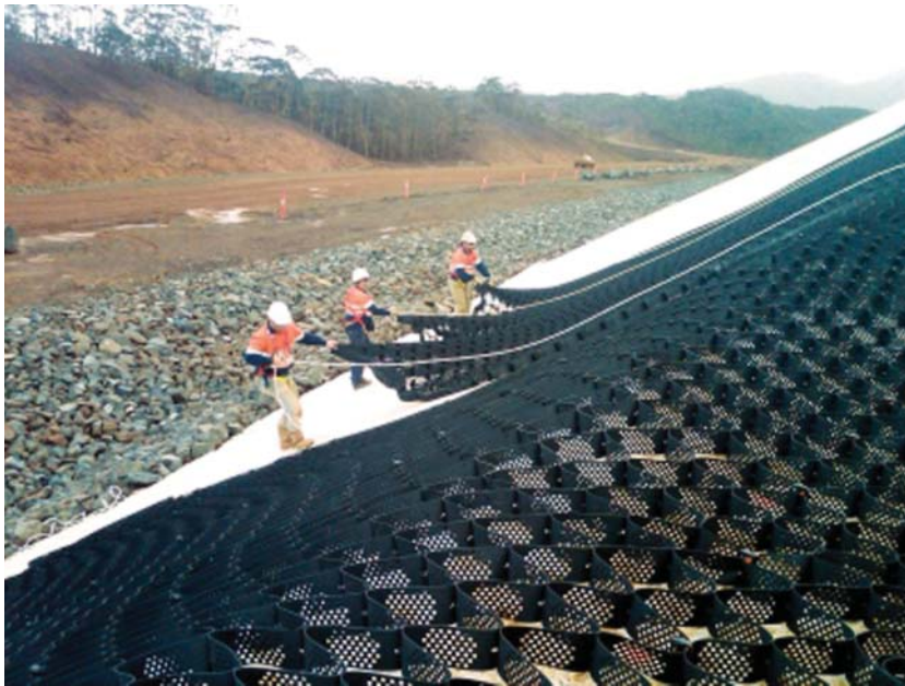
Fig. 6.12 Geocells are placed on the slope surface and then filled with gravel, as a permanent nondegradable erosion control and slope protection layer. (Photo courtesy of Geosynthetics magazine.)
