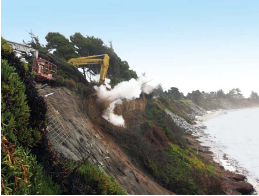
Fig. 7.38 Soil nails are used to stabilize the bluff at Pebble Beach Drive, Crescent City, California. (photo courtesy of Soil Nail Launcher, Inc.)
