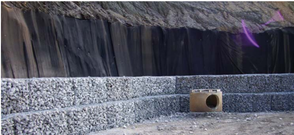
Fig. 8.20 Geotextile filter behind a Gabion basket wall. (Photo courtesy of Midwest Construction Products, Fort Myers, FL.)
