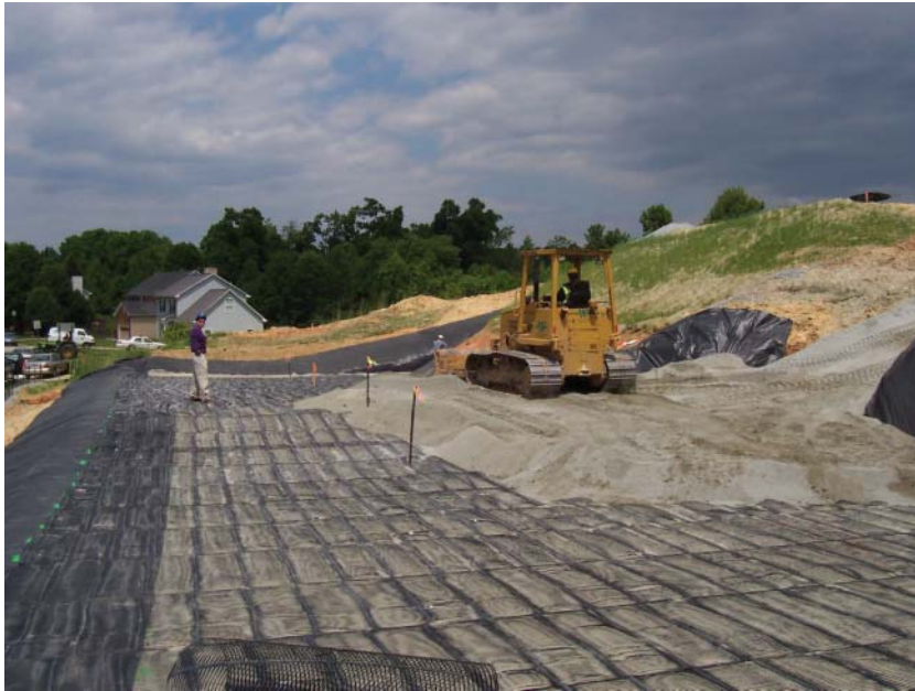
Fig. 5.38 Example of a reinforced soil slope in construction. (Photo courtesy of Tensar International.)
