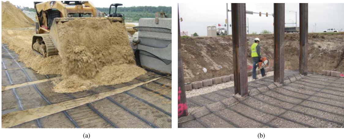
Fig. 8.3 Examples of construction of MSE wall and abutment. (a) MSE wall, (b) MSE bridge abutment. (Photo courtesy of Tensar International.)
