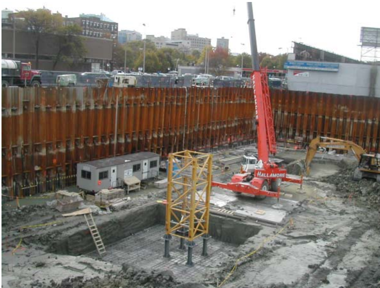
Fig. 7.2 Sheet pile wall for vertical cut. (Photo courtesy of Earthwork Engineering, Inc. Hollis, New Hampshire.)
