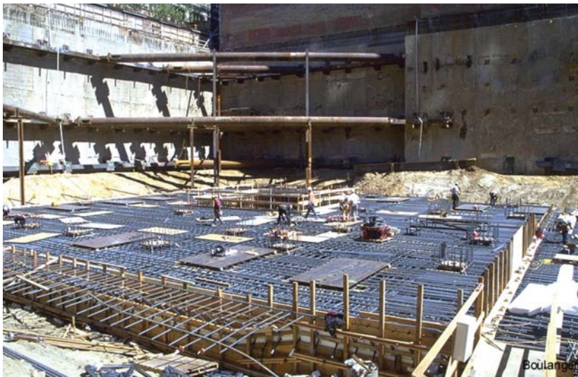
Fig. 3.15 Mat foundation of the Four Seasons Hotel, San Francisco, California. (Photo courtesy of Prof. Ross W. Boulangier, University of California, Davis).
