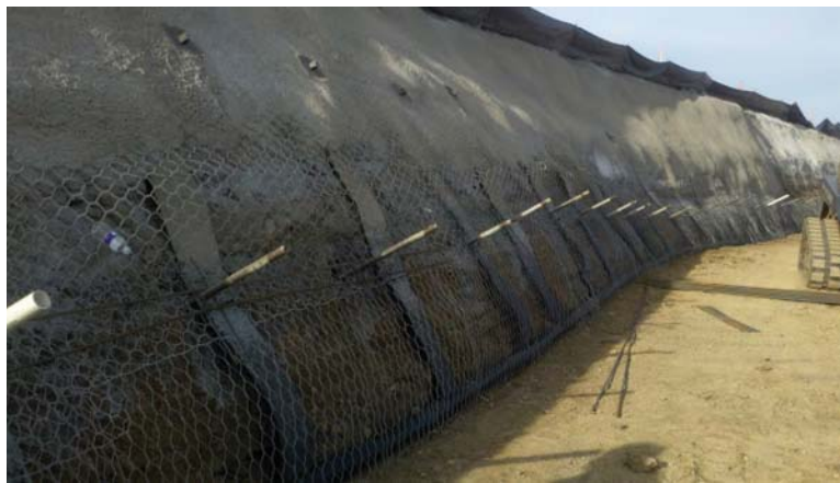
Fig. 7.4 Soil nail wall used to repair a landslide in Montana, USA. (Photo courtesy of Soil Nail Launcher, Inc.)
