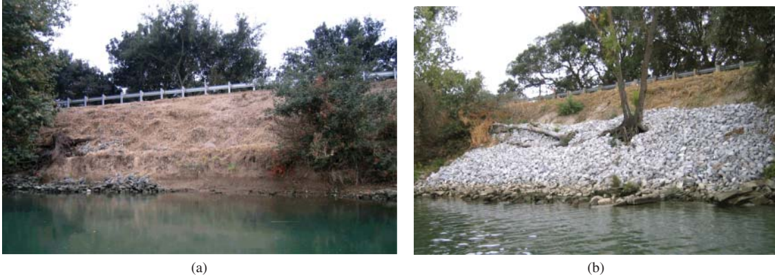
Fig. 6.11 Rock riprap protection of eroded banks of the Sacramento River (California, USA). (a) River bank erosion (critical condition), (b) river bank after rock riprap repair.
